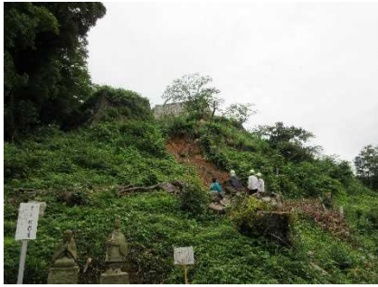
崩落箇所(遠景)
